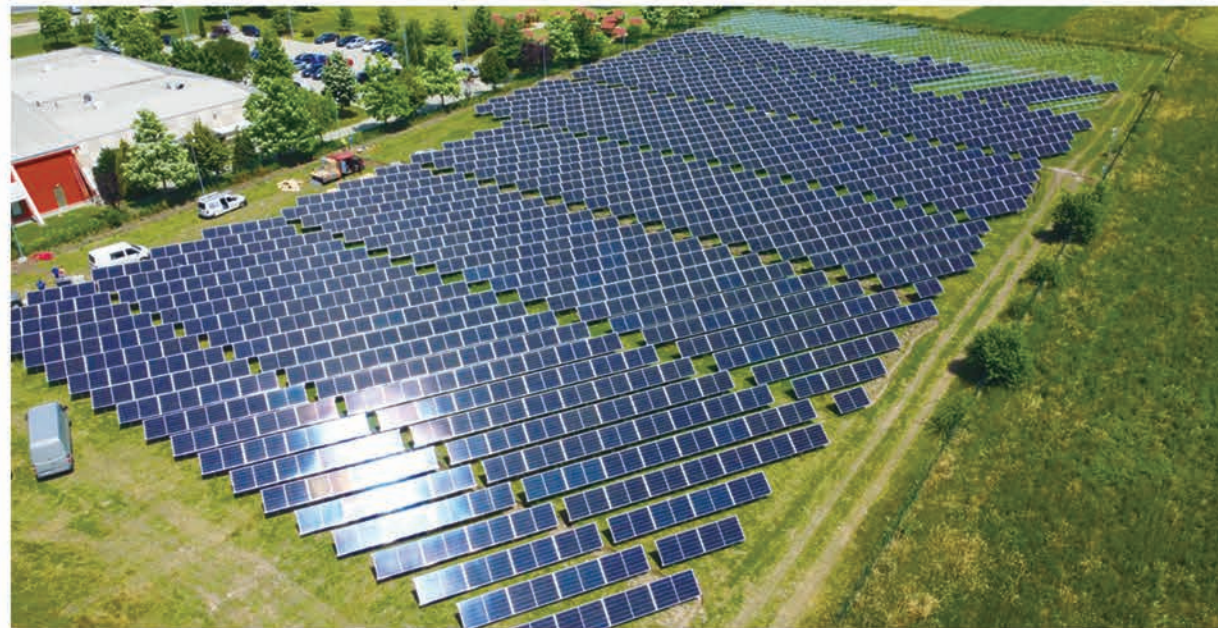
1.1MW PV Power Plant Project of Louisvuitton Plant in Sibiu Province, Romania
