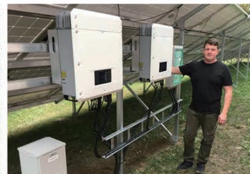
Photovoltaic inverters in European photovoltaic parks project
