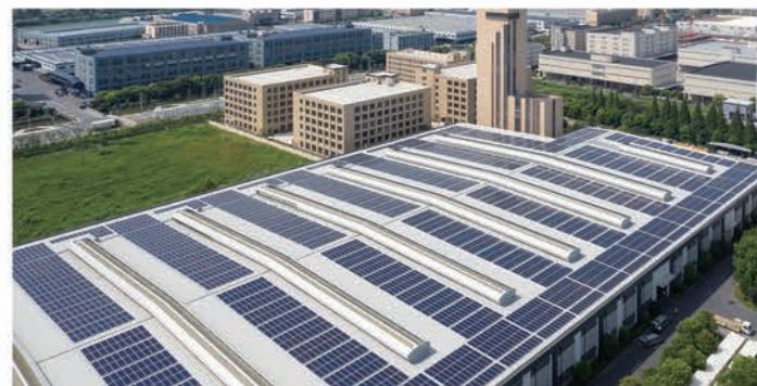
Gansu Tianju power station project 49MW
